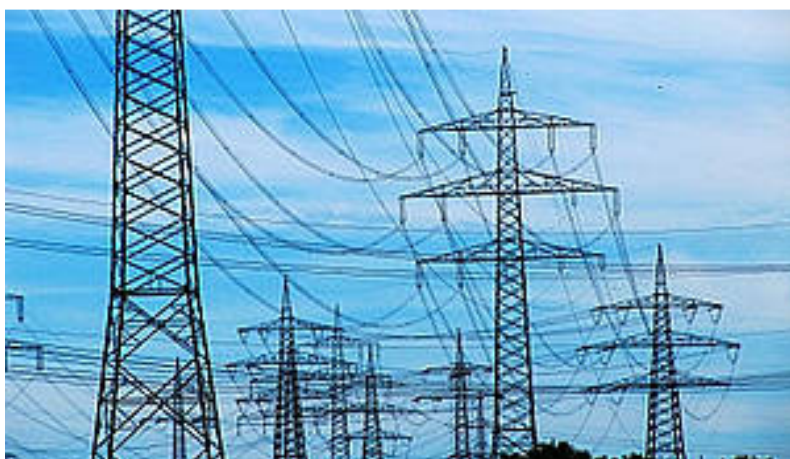
More than just a missing grid. Photo: G. Sturm; Pixelio
